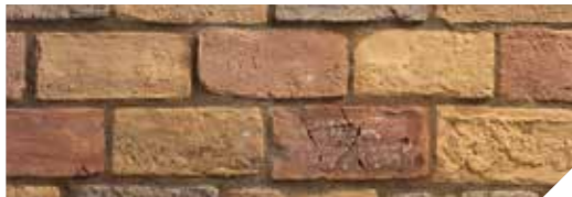
FIRE BRICK INTERIOR
